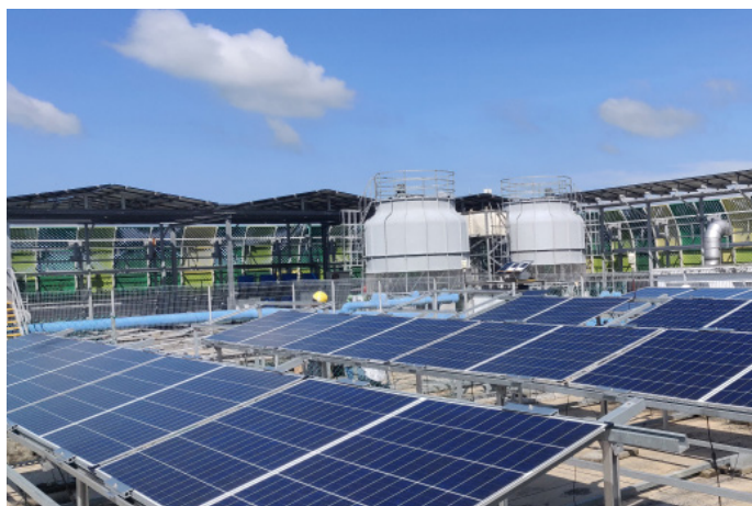
SERIS' rooftop facilities at Clean Tech Park
